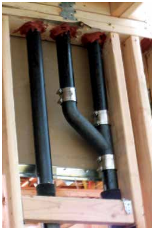
Plumbing joints with pipes nested in joint to allow for vertical movement of structure
